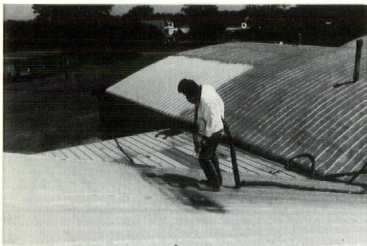
Our Urethane roof system being installed at 1800 S.W. 2nd St., Des Moines, Iowa.
