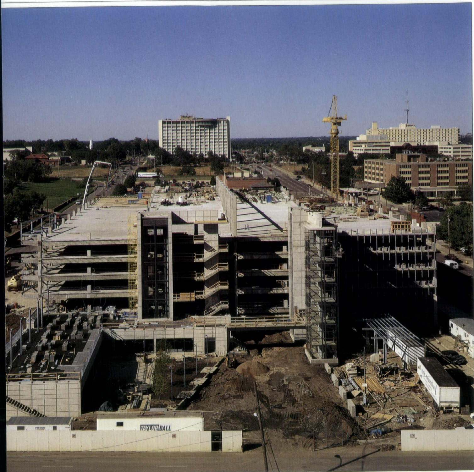
Above: The construction photo of Intermodal's south facade shows how the architect detailed concrete to accommodate the many requirements of the structure.
