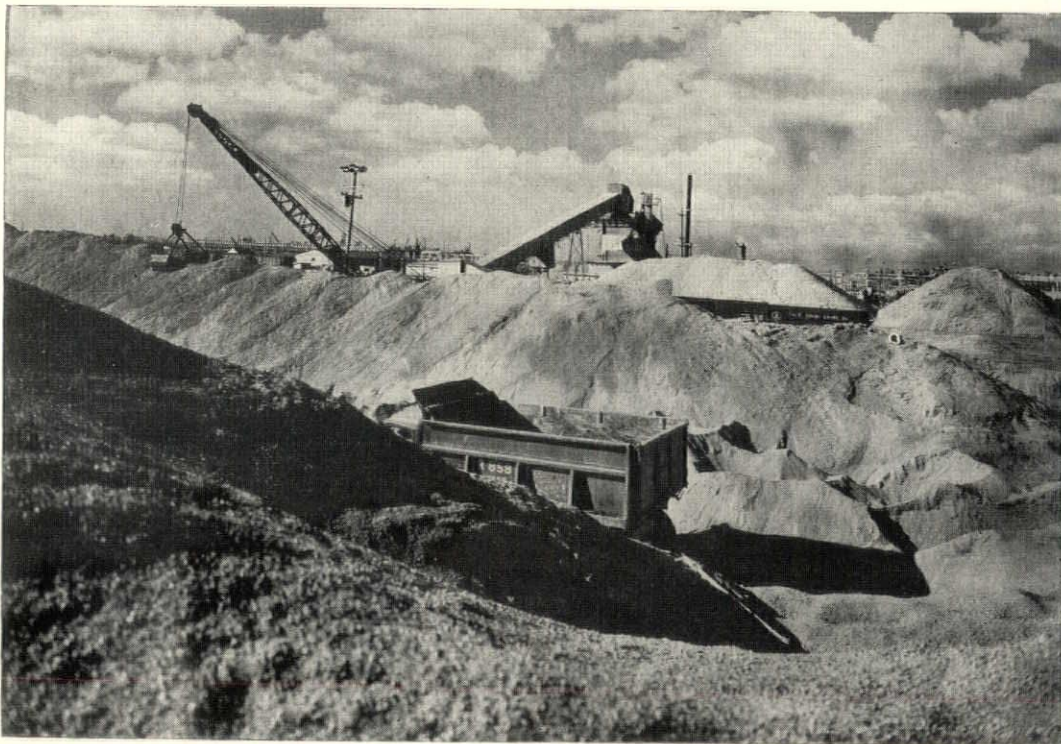
ONE HUNDRED FIFTY CAR LOADS of sand, cement and stone are brought into the Dodge Chicago Plant every day for construction work. In the background of this picture can be seen one of the two concrete mixing mills which were built on the plant property for this construction job alone.
