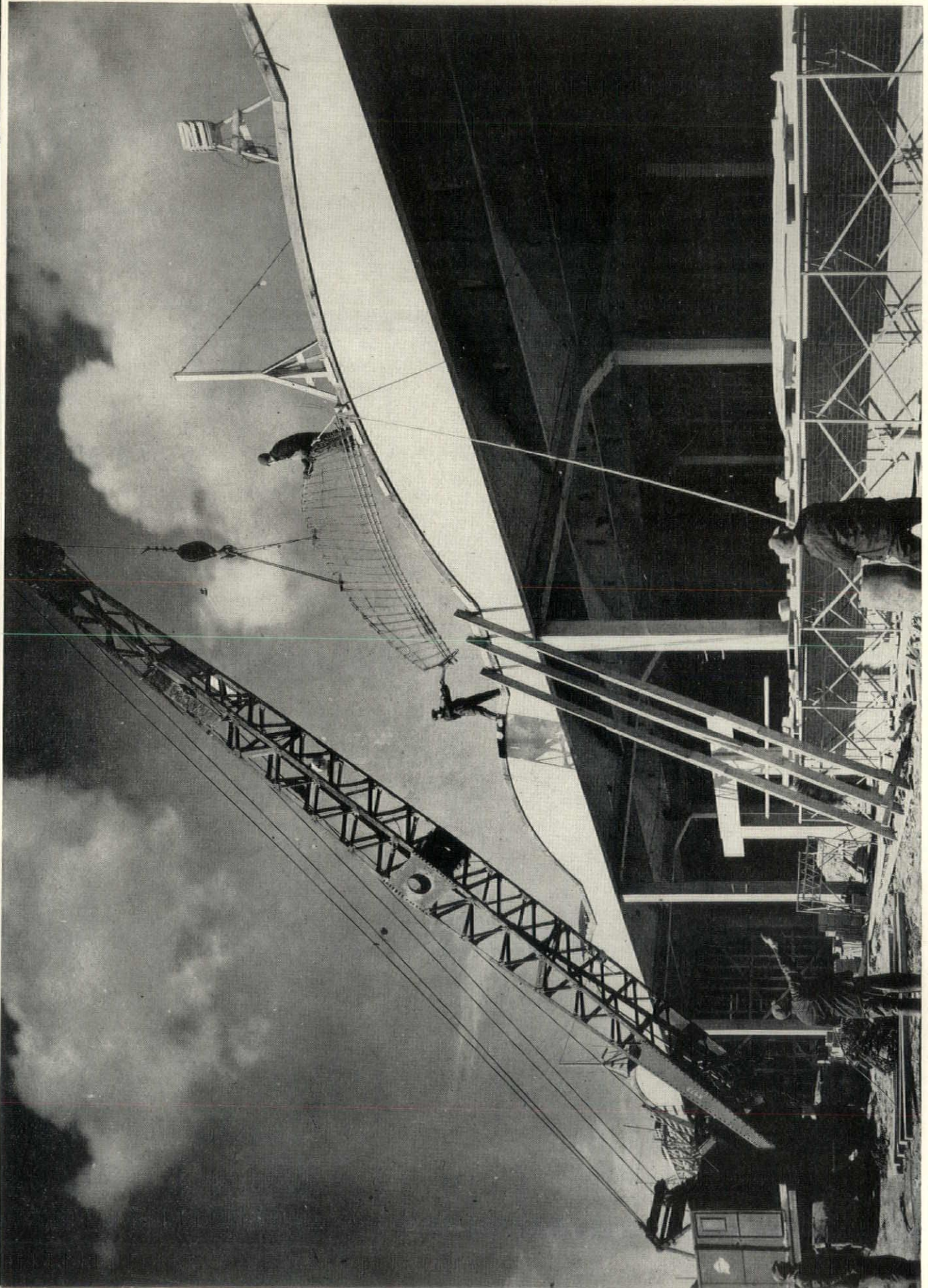
FIFTY CITY BLOCKS UNDER ONE ROOF—that will be the size of this building which will be one of fifteen in Chrysler Corporation's new Dodge Chicago Plant. When it is finished most of it will be fresh-air ventilated, but one small section of 22 acres will be completely air conditioned.
