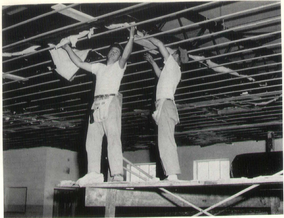
Above shows an application of cotton blanket insulation on a suspended ceiling in an industrial building.
