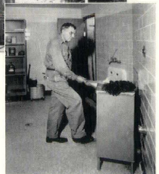
Dry mops are vacuum cleaned at Mop-Vac cabinet connected to Spencer central vacuum cleaning system.
