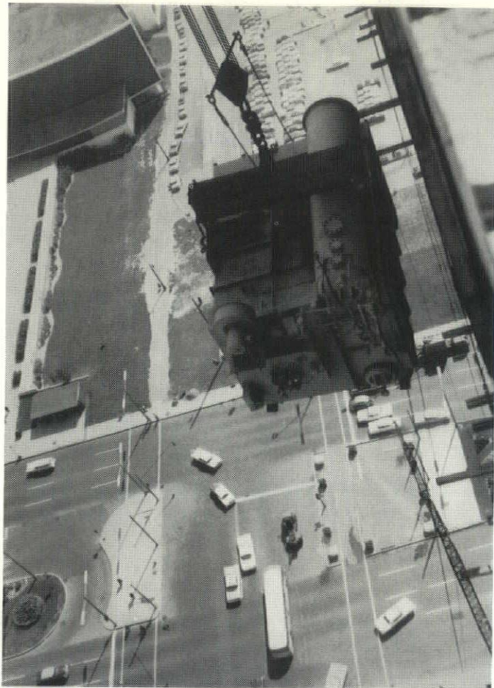
◀ 27-ton boiler on its way to the top of Gas Company building where it was joined by another boiler and the air conditioning equipment.
