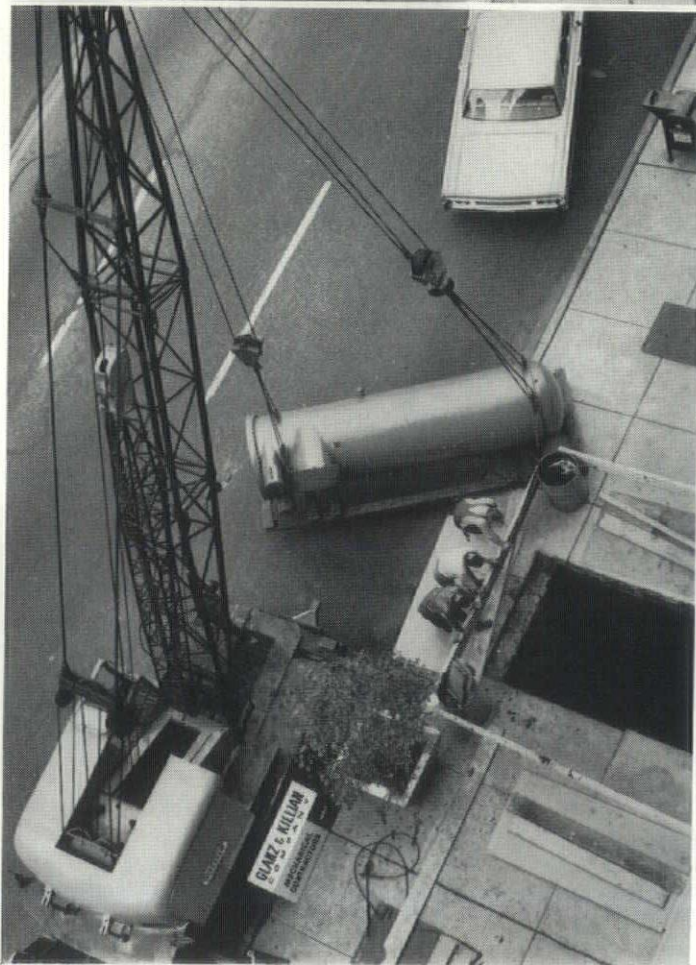
◀ One of two Chrysler AIRTEMP centrifugal water chillers on its way to the new air conditioning system in the basement of the Federal Building.
