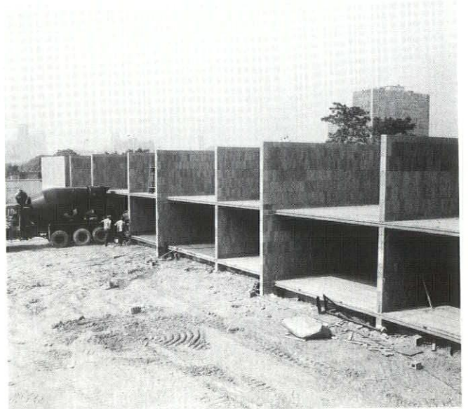
Early construction at the Martin Luther King, Jr. homes in Detroit showing walls of concrete block constructed with Threadline brand adhesive mortar. The current project involves 58 buildings containing 480 living units.
