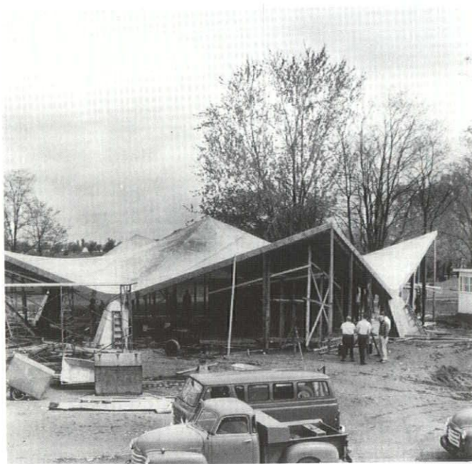
Thin shell construction in service station at Midland utilizing Styrofoam for the hyperbolic paraboloid roof.
