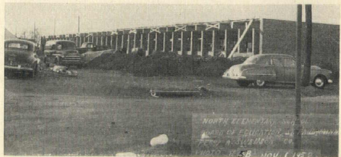
In North Elementary School (above) architects used a combination of laminated wood beams resting on masonry bearing wall which on the window wall become brick piers. Construction avoids use of any steel, although cubage costs for this structure equal those for similar schools erected in this program of steel frame.
