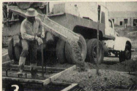
3 Place concrete, using quality mix yielding durable walls. Use care to prevent honeycombing, especially along bottom edge.
