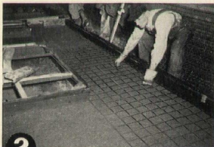
2 Place the required amount of reinforcing in the panel and be sure to provide suitable means to hold it in the proper position.
