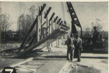
7 With crane or hoist tilt the panels into position in wall. Grout joint between the wall and the floor to make it weathertight.
