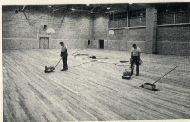
Finishing with a wood seal buffed into wood by steel wool machine.
