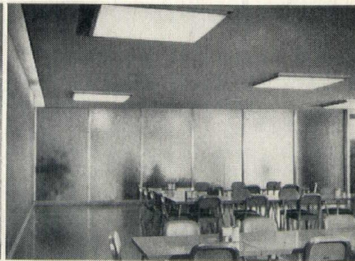
In the Central Exchange building lunchroom, Crown fabricated the extruded aluminum air diffusers around the light fixtures, the aluminum partition framing and all the stainless steel aisle railings.
