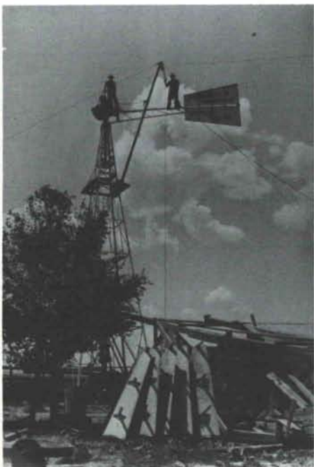
Use of a gin pole to lift windmill components to the top of a tower. Courtesy B. H. Burdick, Sr., and Panhandle-Plains Historical Museum, Canyon, Texas.
