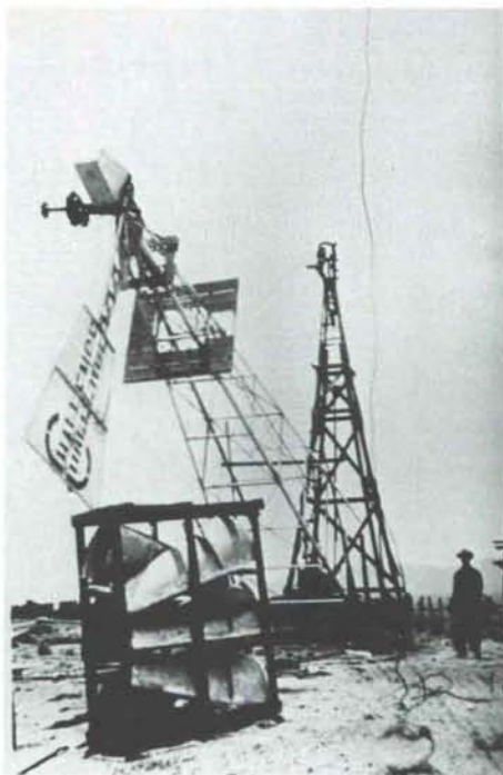
Raising a steel tower with large "Challenge 27" windmill in southern New Mexico half a century ago. Courtesy B. H. Burdick, Sr., and Panhandle-Plains Historical Museum, Canyon, Texas.
