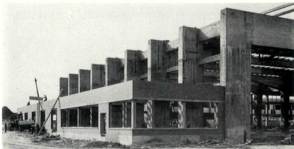
Construction Photograph of West Side of Hangar Showing One Story Office Section
