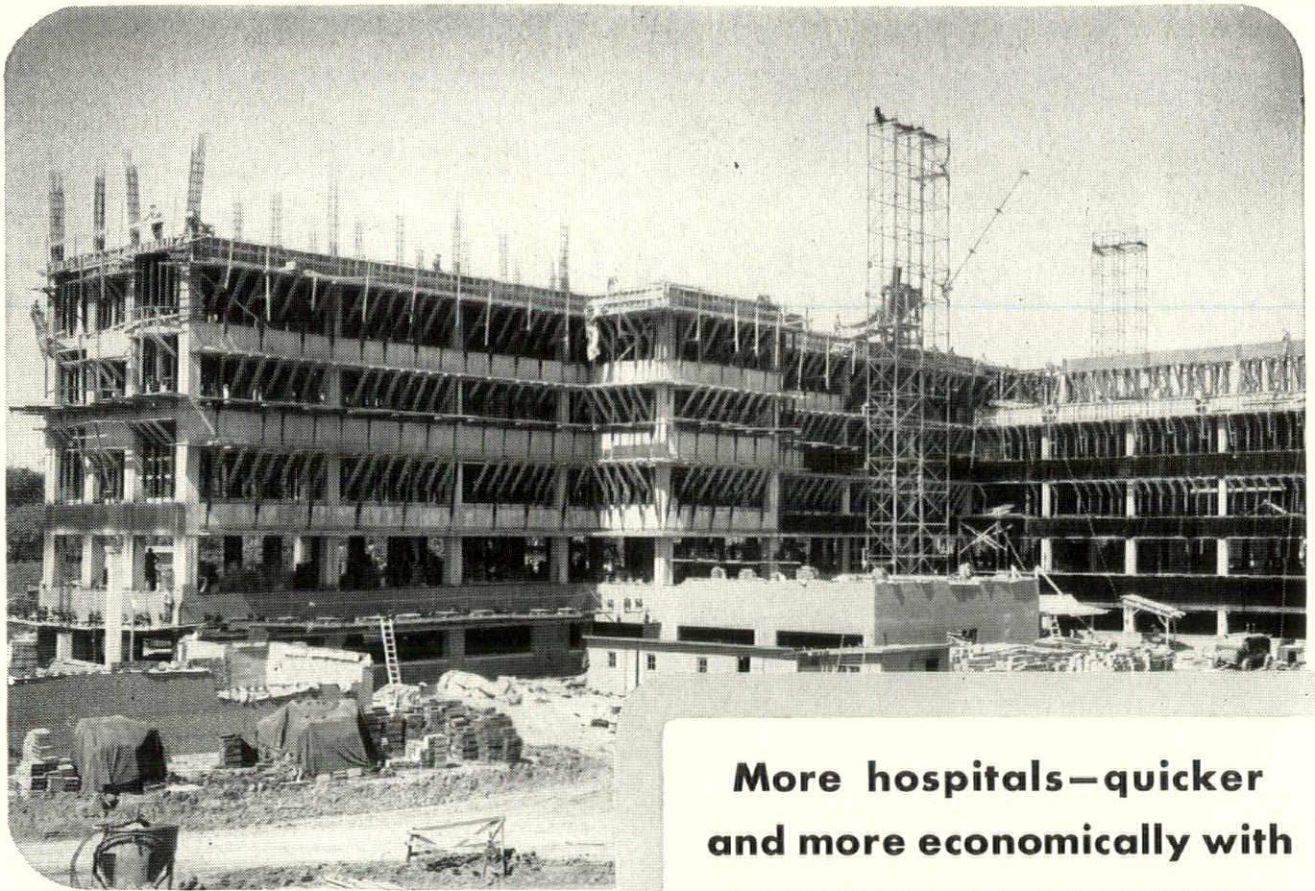
Construction view of 10-story, 500-bed Veterans Administration Hospital, Iowa City, Iowa. Ellerbe & Co., St. Paul and Leo A. Daly Co., Omaha, architects and engineers. Gust K. Newberg Construction Co., Chicago, general contractor.
