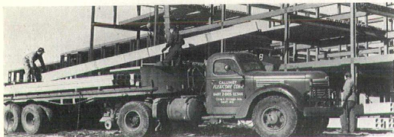
Long-span Flexicore slabs are trucked to site as needed. Floor and roof construction proceeds in freezing weather. No forms for pouring of concrete necessary.
