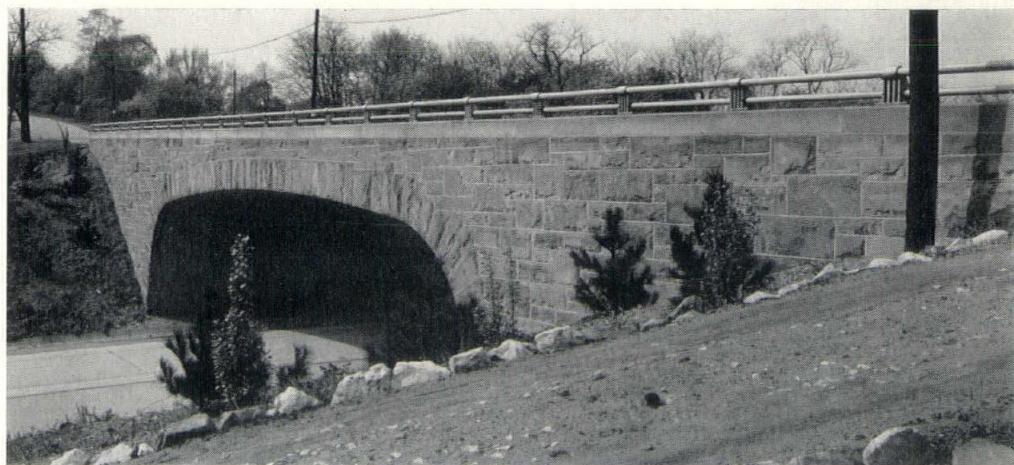
Penn-Lincoln Parkway, Greensburg Pike Bridge Johnson-Drake & Piper, Contractors Dept. of Highways, Architects & Engineers
