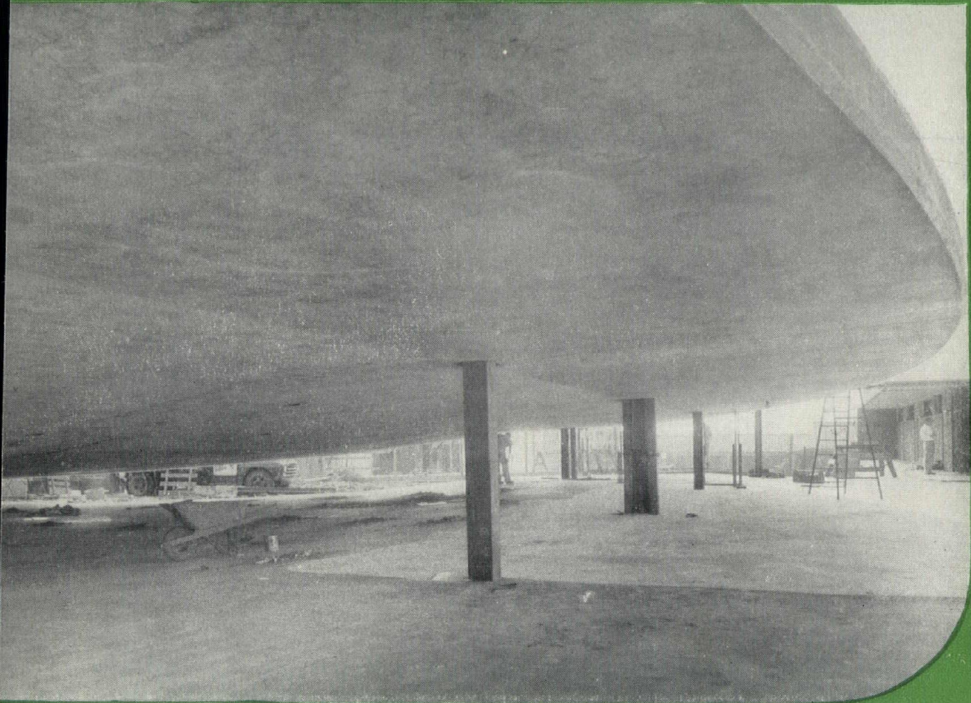
A million pounds of concrete slab practically "floating in air." This picture shows the concrete roof slab of the New Temple Isaiah of Los Angeles being raised into place. See story on page 10.
