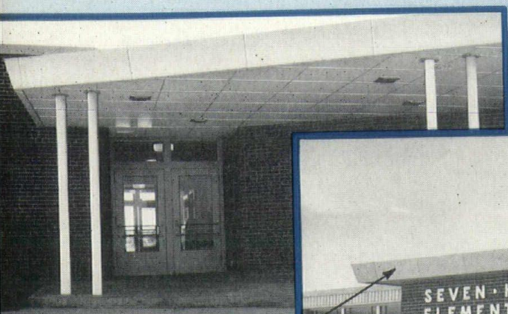
◀ The clean lines of this one-floor design are emphasized by the Davidson Architectural Porcelain used on the canopy and gravel stop pictured here.
