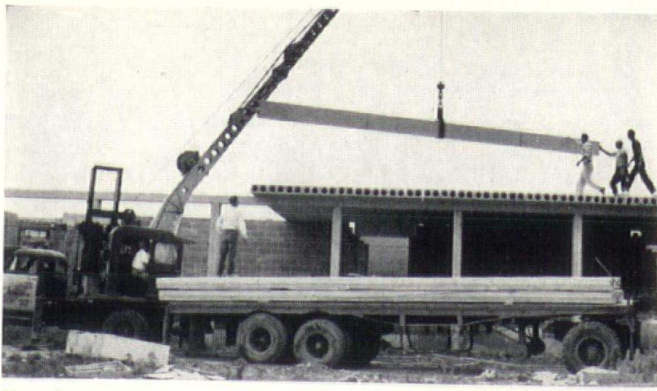
Firesafe concrete roof is erected in a few days. Flexicore roof slabs are precast in factory, keep costs low, save on-the-job labor.
