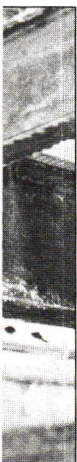
Joining new steel to old was a challenge for engineers at George M. Levinson, as they designed the structural support for the First & Market renovations.
