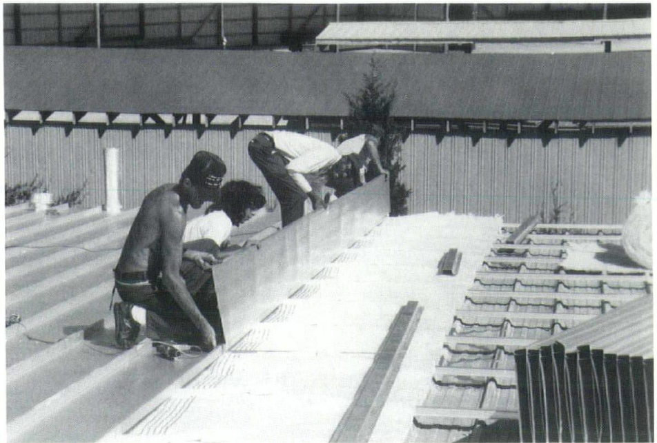
Working in phases, it took Henley Roofing Co. 27 working days to complete the metal roof retrofit with crews of five to eight men.
