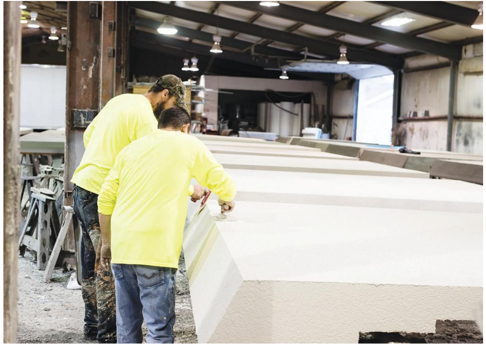
Fabricating EIFS panels indoors avoids the problems of weather and scheduling delays often associated with field construction.
