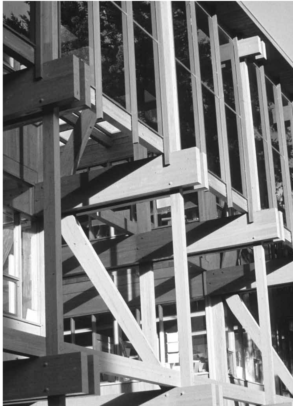
Details of by-pass wood construction and diagonal struts that resist wind and seismic forces eliminating the need for interior shear walls. Image from the Visual Resources Collection, College of Built Environments, University of Washington.
