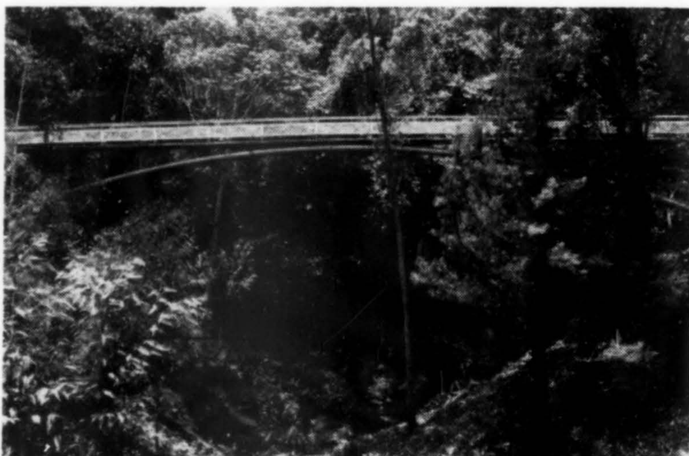
RED STEEL FOOTBRIDGE is located in the Botanical Gardens, Honolulu, approaching Schofield Barracks. George Lee was bridge architect.
