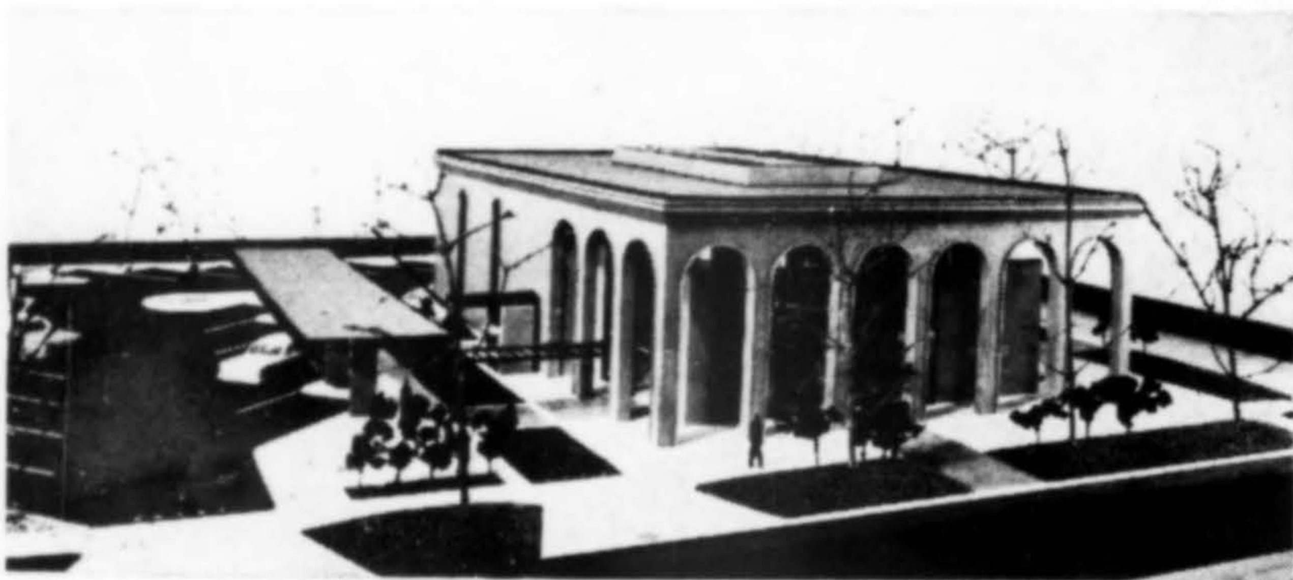
CONSTRUCTION has started on the First Federal Savings & Loan Association's new building in Salem, Oregon. Exterior will be amber rose-red brick with dull bronze anodized aluminum spandrels, windows and doors, grey solar glass. Masonry arches, projecting corbelled parapets and brick arcades on three sides of the two-story building provide pedestrian shelter and solar control in summer. Landscaping includes Gingko trees on two street fronts with benches surrounding circular pool and fountain. Architects: Wilmsen, Endicott and Unthank, Eugene and Portland; Mills Construction Co., Salem, contractor.
