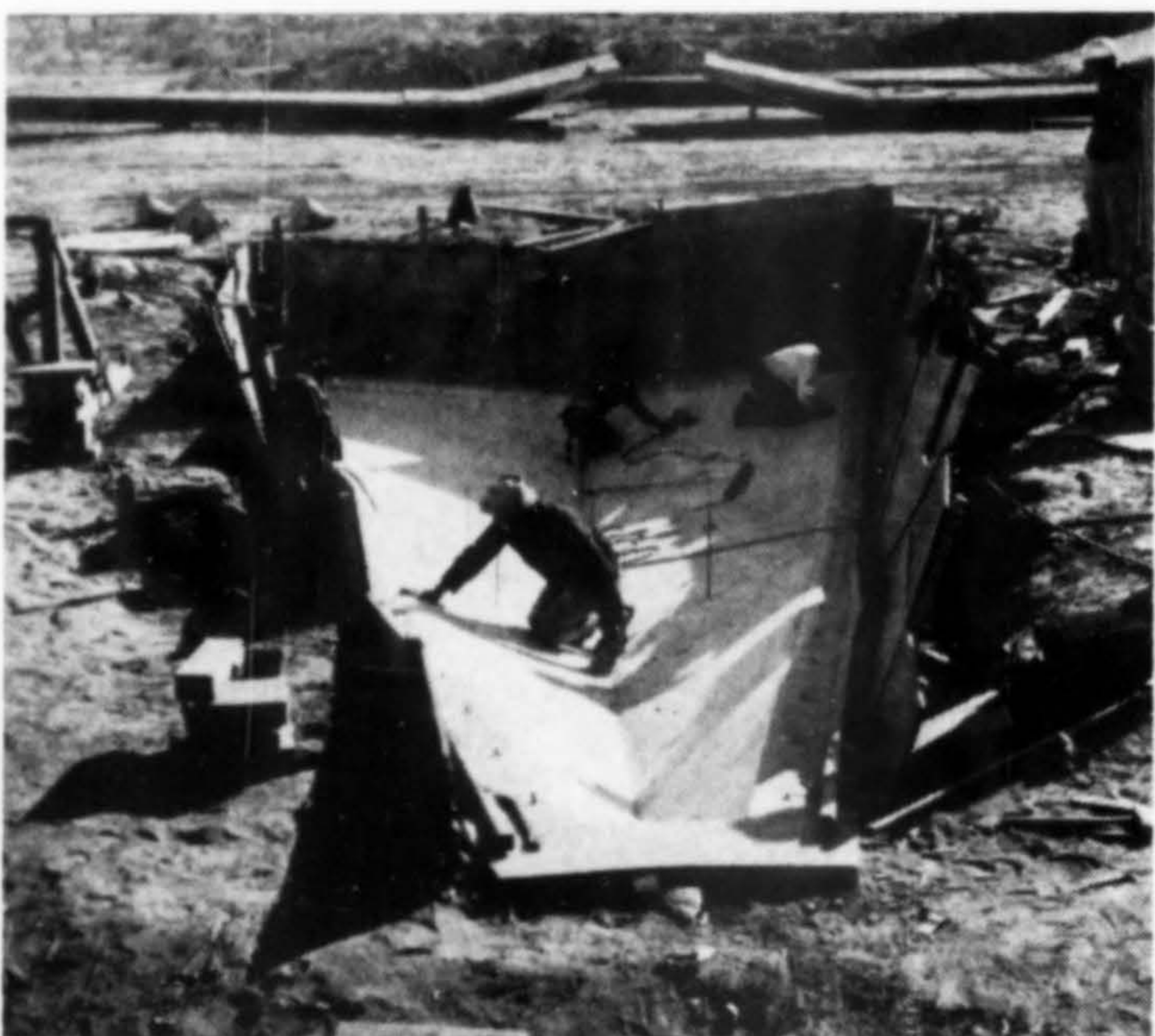
In precasting the 16 roof segments, the ground was sloped and shaped to give final position of the concrete form. Concrete was job-mixed using special plasterer's sand and the surface was then steel troweled for a dense, smooth finish.
