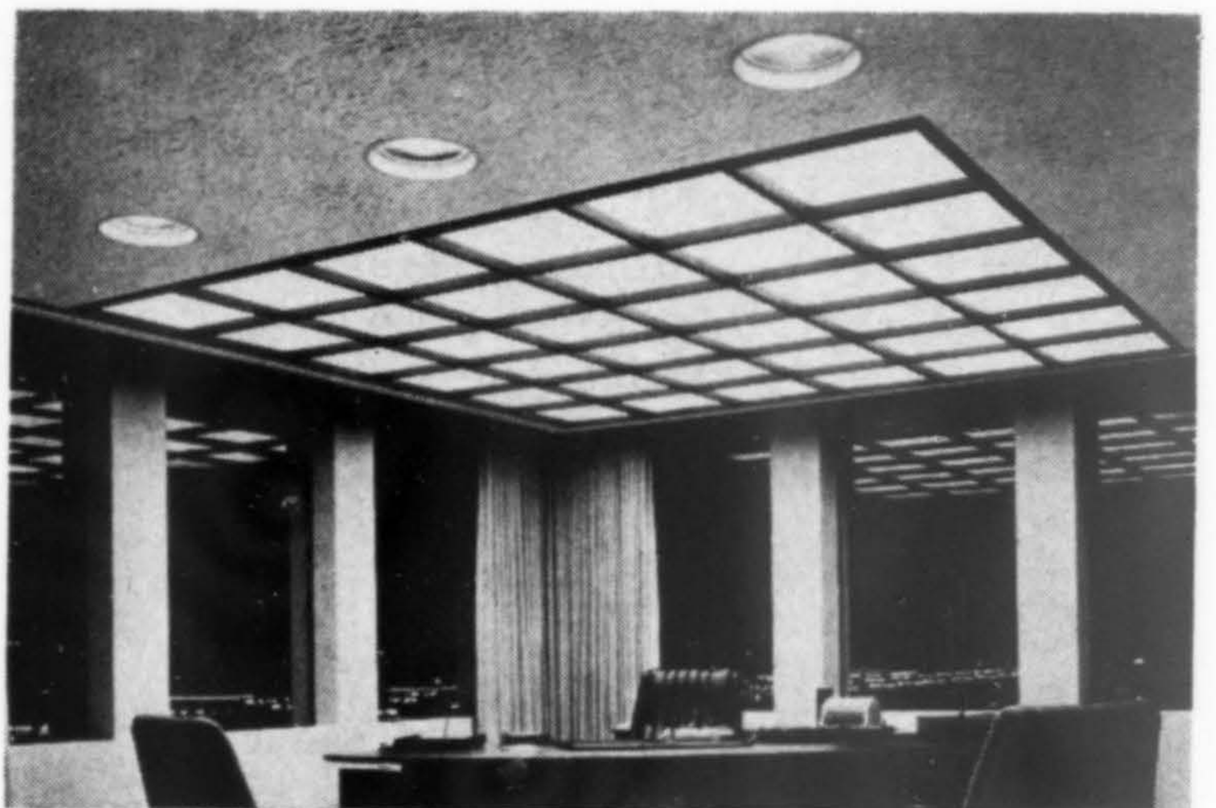
Two different lighted ceiling systems were installed in the overhead area of the executive offices of the United Financial Savings & Loan Association (Welton Becket & Associates, architects). They provide a fluorescent lighting contrast to surrounding incandescent downlights. Each system is also controlled by separate switching to permit different effects, keyed to function and mood. A "Lightframe" system fills 150 sq. ft. of the overhead area and a "Heritage" system occupies 70 sq. ft.
