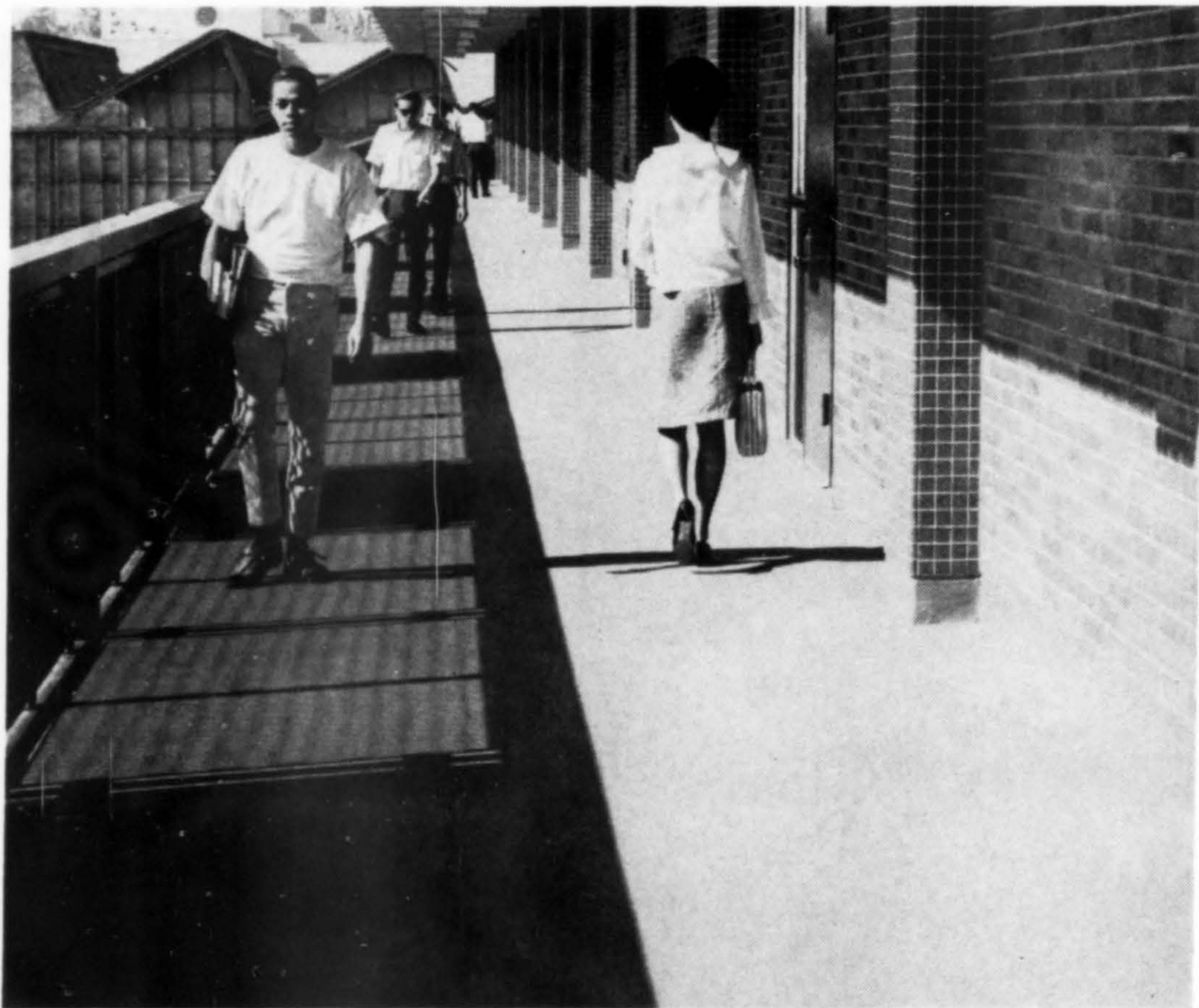
Technology Bldg., Pasadena City College, Pasadena, Calif. Architects: Allison & Rible. Applicator: Owen Roofing Co., Los Angeles.
