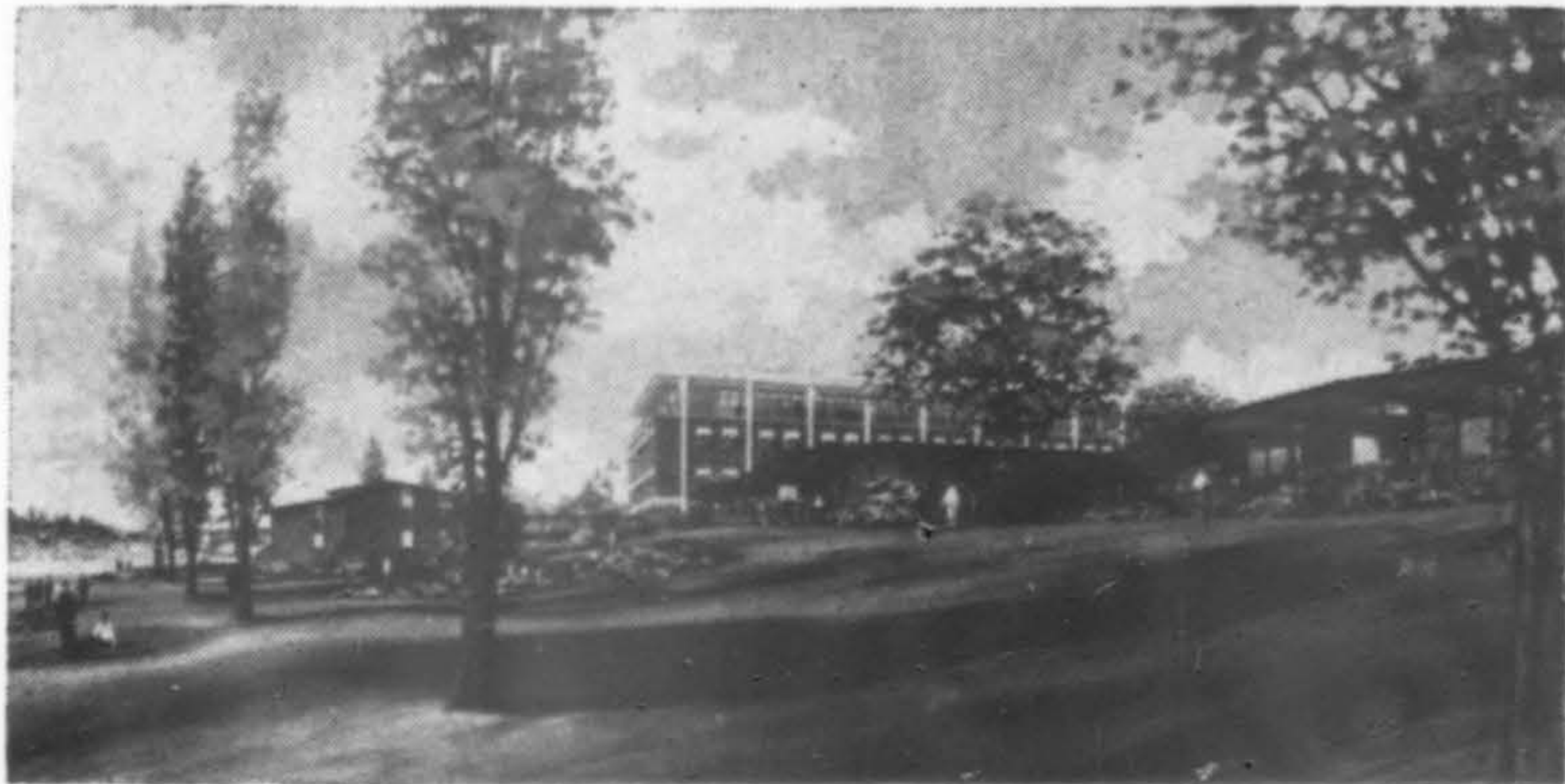
FINAL construction phase of the Center for Research and Training in Mental Retardation and Child Development at the University of Washington, Seattle, will consist of a four-story Diagnostic Clinic, a one-story Laboratory School and a two-story Short-Term residence unit. Estimated cost: $4 million. Architect: Arnold Gangnes.
