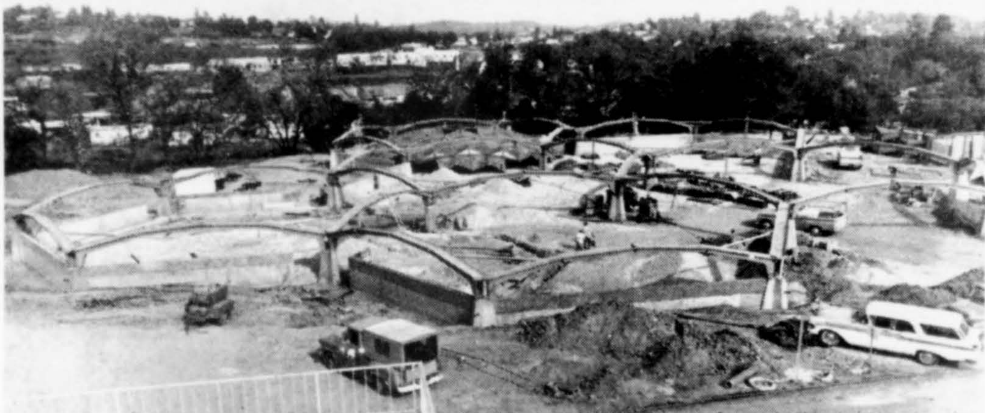
Rings which support the aluminum geodesic domes are in place and the first of six domes is being erected.
