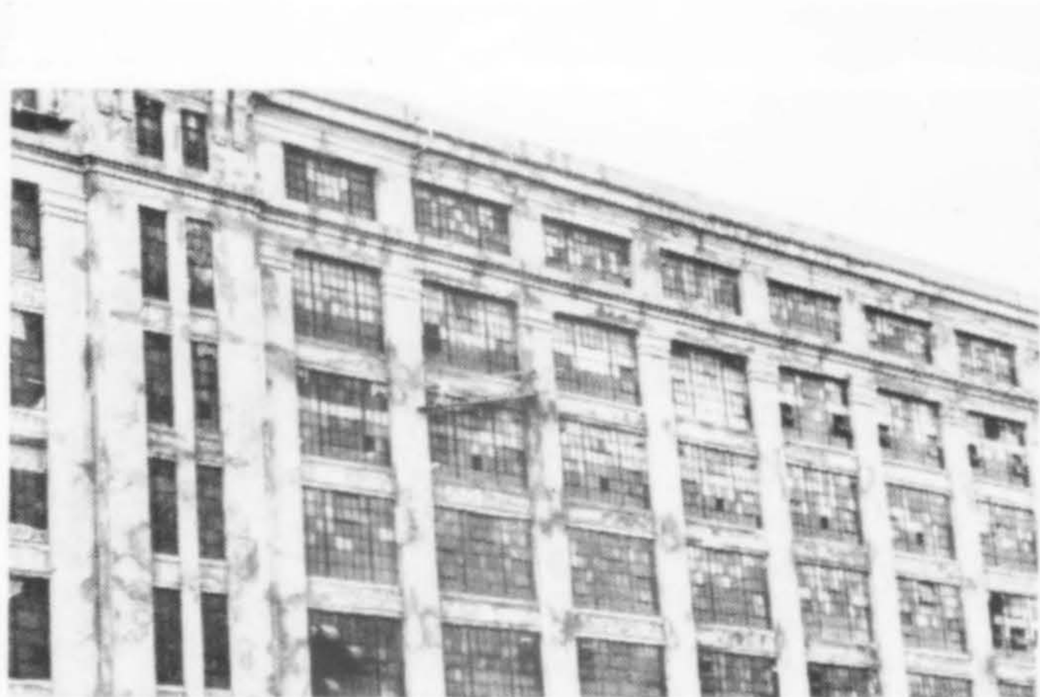
Exterior concrete on building at Boston Army Base has deteriorated badly . . .
