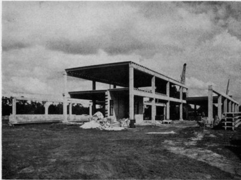
T. G. LEE DAIRY under construction in Orlando. Roof slabs, floor slabs, beams, and columns are all prestressed precast concrete . . . furnished by Holloway Concrete Products Co. of Winter Park, Fla. Charles Johnson, Architect . . . E. M. Scott, Contractor . . . Lakeland Engineering Associates, Inc., Prestressing Consultants. Double Tee roof spans vary from 36 to 40 feet. The beams and columns are hollow. Of special interest is the two-story column cast in one piece.
