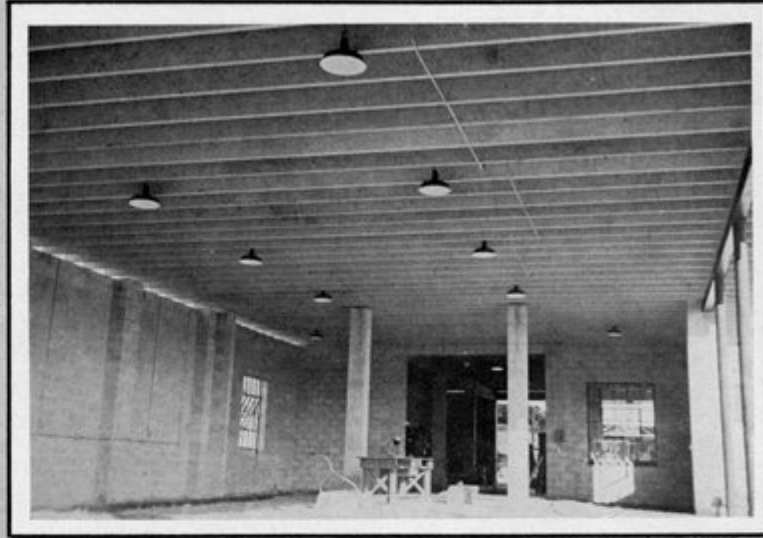
40' span prestressed concrete Double tee garage roof deck at Holloway Concrete Products Co., Winter Park, Florida.
