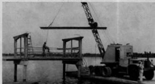
How to build a dock quickly at low cost is illustrated in this scene at Lakeland. Crane is resting on dock of LEAP Double Tees, hoisting 30-foot roof slabs!
