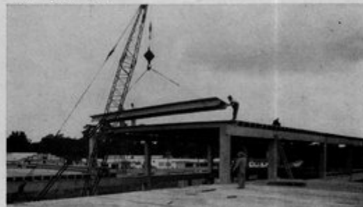
Construction scene at the new T. G. Lee Dairy, Orlando. Crane is lifting 38-foot LEAP Double Tee roof slabs into place in this modern structure.
