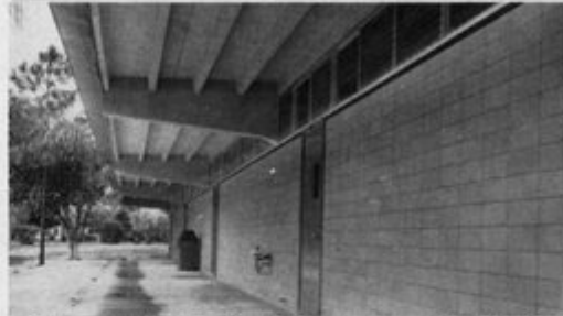
Exterior corridor at the Stuart, Fla., elementary school, showing use of LEAP Double Tees supported on a cantilevered concrete rigid frame.
