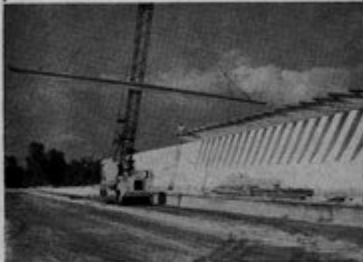
LEAP Pre-Stressed concrete tee joists in this Mayflower warehouse give long, clear spans with no truss supports or posts to take up valuable space.
