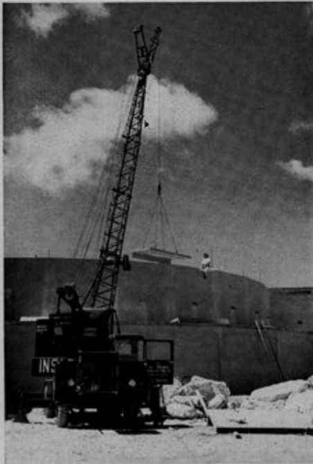
Precast concrete slabs being hoisted to top deck for tiered standing platform.
