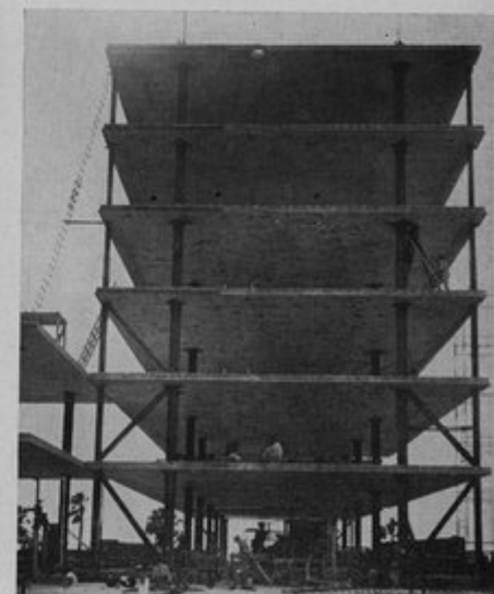
All slabs were lifted and permanently anchored in place within five weeks.
