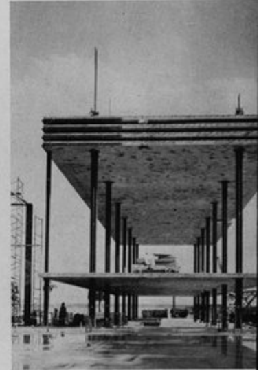
Lower floor slabs were next lifted permanent levels and anchored in place.
