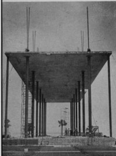
All slabs were poured on the ground and the first one lifted was 14 days old.
