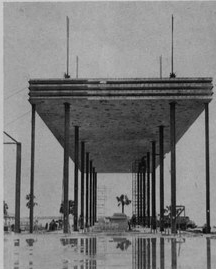
Slabs for roof and three upper floors were lifted first in temporary positions.
