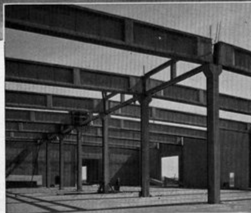
Top photo: general view of warehouse at Long Beach, Calif. Exterior longitudinal walls are precast concrete panels 30-ft. high, 23-ft. wide and 6 in. to 8 in. thick. Photo above shows 56 in. deep, I-shaped girders supported on cast-in-place wall columns and precast interior columns. Span of the precast girders is 75 ft.
