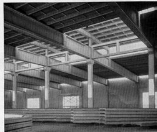
Roof constructed of precast concrete channel slabs resting on prestressed girders and precast monitor frames. Warehouse designed by the office of the late J. H. Davies, consulting structural engineer. Structural engineer was James R. Bole of Long Beach, Calif. Contractor was Johnson-Western Constructors of San Pedro, Calif.
