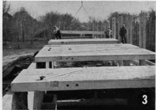
3 After rear walls were brought to second floor elevation, 3-ft. wide precast concrete floor channels with 10-in. legs were placed across the entire width of the buildings. Below is a view of the underside of the floor showing how conduits pass through sleeves in the legs.
