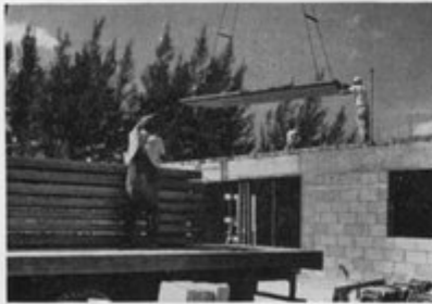
Slabs can be erected at rate of 8,000 sq. ft. per day. Tongue and grooved edges speed placement, give greater stability. Undersurface is smooth, ready to paint or plaster.
