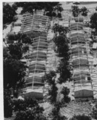
Elementary School Project "C" Vero Beach, Fla. Rilco laminated pitched beams spans 36, 40 and 56'. Architect, David V. Robinson, Vero Beach. Contractor, Clutter Const. Corp., Miami Springs.
