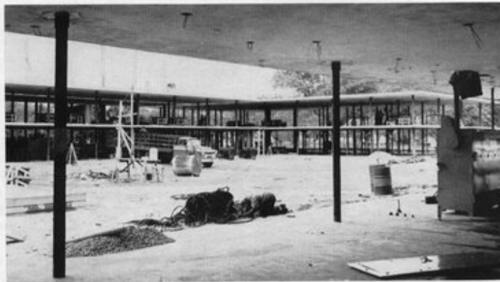
One result of the lift slab method of construction was accurate placement of sleeves for utility lines and ducts, together with structural precision making possible use of pre-cut materials to conserve job time and labor.
