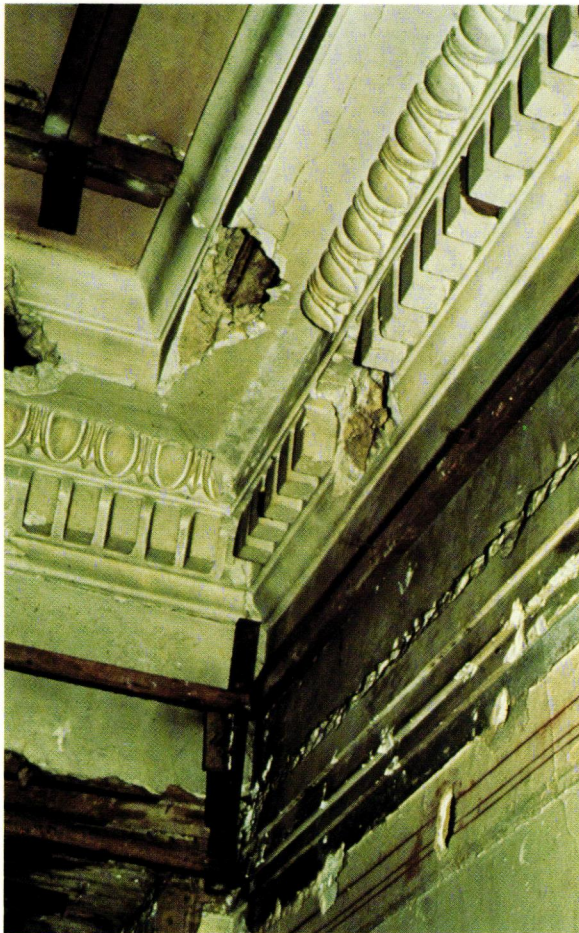
Detail showing deteriorated section of interior moulding prior to restoration. Photo by Catherine D. Lee, AIA.
