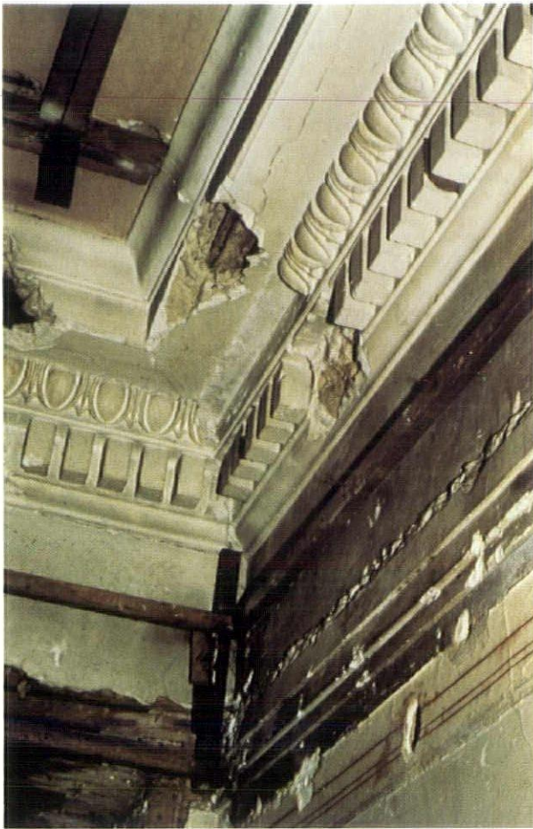
Detail showing deteriorated section of interior moulding prior to restoration. Photo by Catherine D. Lee, AIA.
