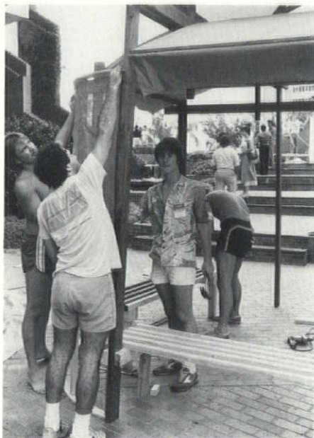
University of Florida Juniors put the finishing touches on the winning shelter at the Student Design/Build Competition in Tampa.
