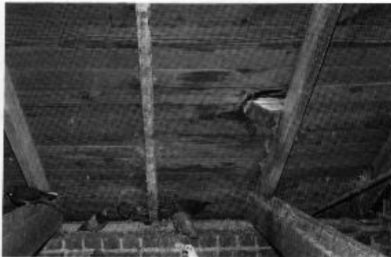
Note deteriorated roof timbers which allowed pigeons to gain entry to the attic area of the building under restoration. Photo by Leroy Gray.
