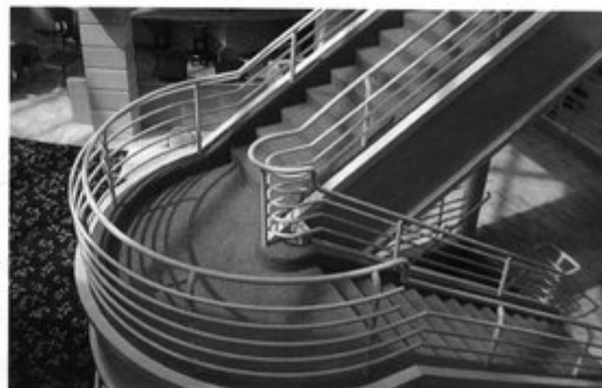
This ornamental stairway is an example of a good design that meets standards and retains its aesthetic appeal. Photo by Randy Atlas.
