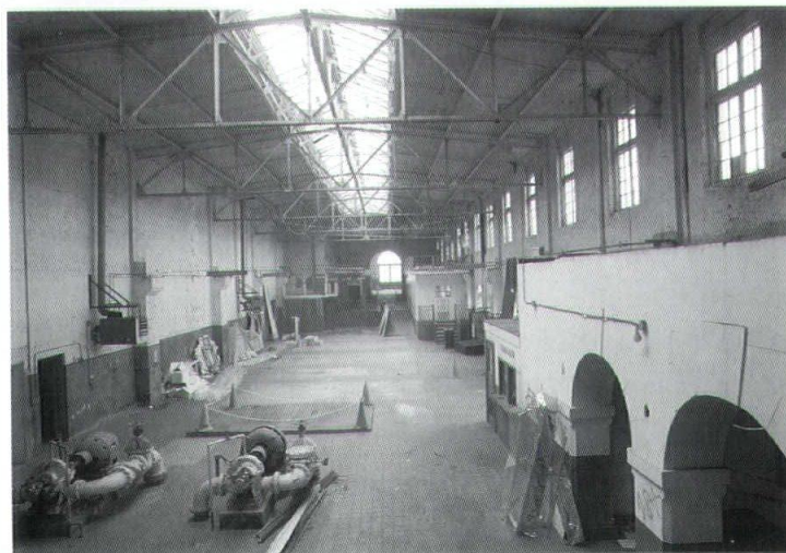
This page, top, renovated exterior of original Orlando Utilities Commission Building which is now home to the Performing Arts Center. Inset shows facade detail. Above, interior of pump room prior to renovation. Photos by Bob Braun. Opposite page, sections through north and west sides showing new internal spatial arrangement. Drawings courtesy of the architect.
