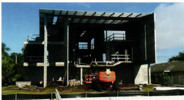
The Nestor Residence is Halflants + Pichette's first design-build project. On the bay side, the roof extends 30 feet beyond the conditioned enclosure. The large overhanging plane folds down to become a wing wall, shielding a distant power plant from view.
