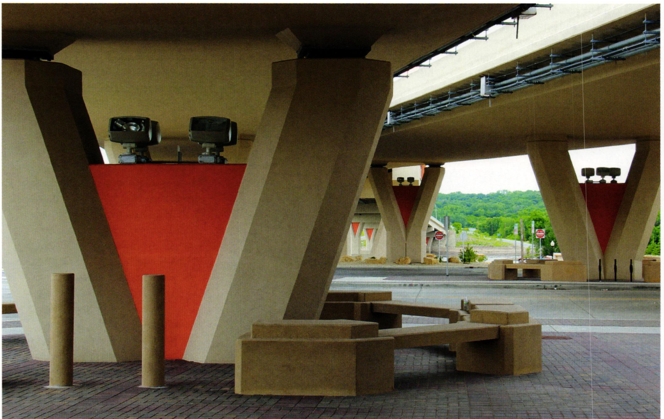
Detail of one of the bridge plaza piers showing collision barriers that double as seating.
