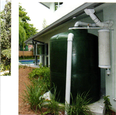
Sustainable elements include a 1000-gallon rainwater collection bank, two solar-thermal panels for hot water, a solar-thermal pool heating system and insulated concrete forms, minus the foam insulation on the outside to minimize cracking during a potential hurricane.
