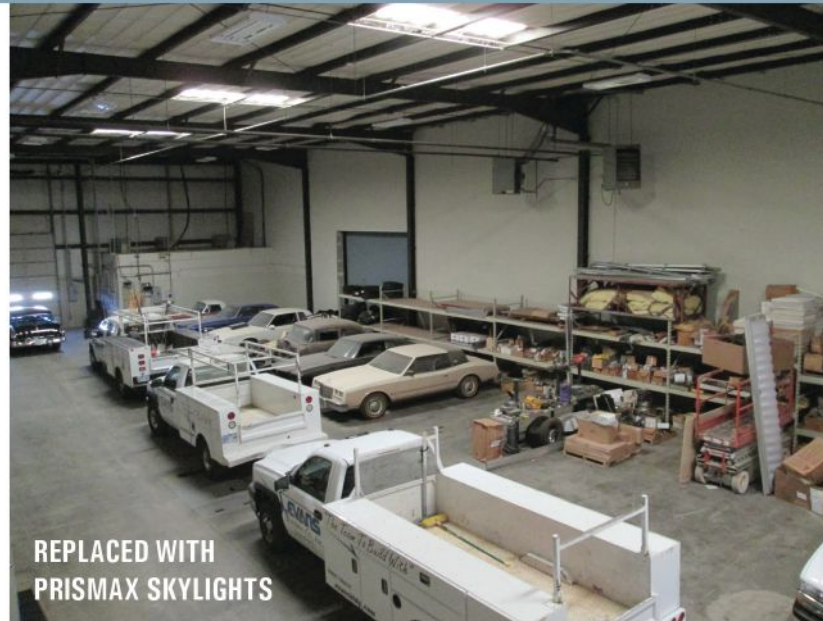
OLD TRANSLUCENT SKYLIGHT PANELS
